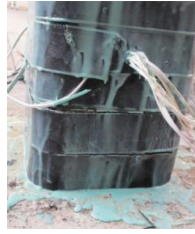
图 8 纤维带之间开裂 Fig. 8 Cracking between fiber belt
