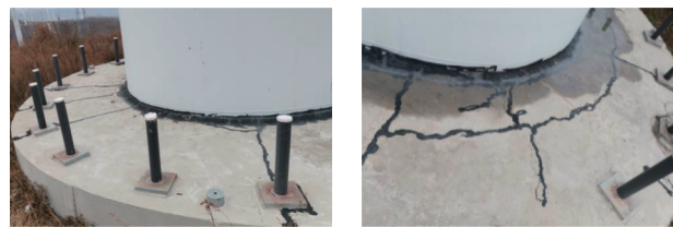
(a) 径向裂缝
